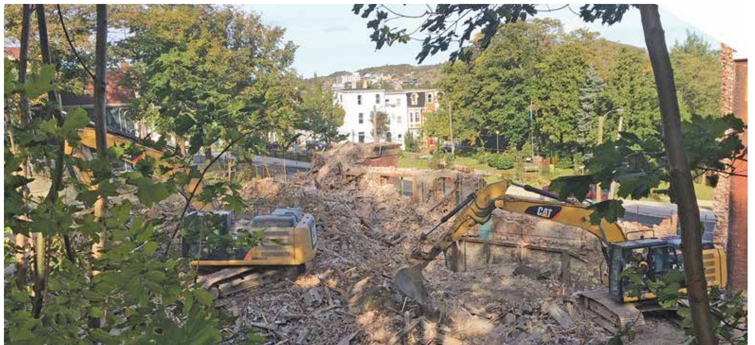
The photographs on this page show the parish hall at various stages of being torn down. The top one was taken by the Rev'd Fred Marshall, and the other two were taken by Ellen Reid.
